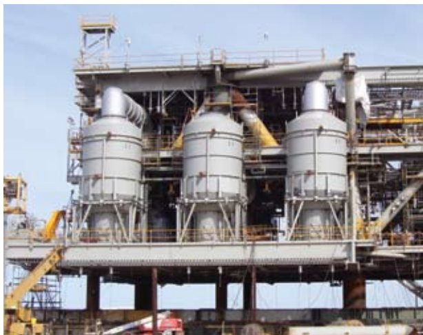
CiBAS units installed at Chevron's Tahiti field in the Gulf of Mexico.
