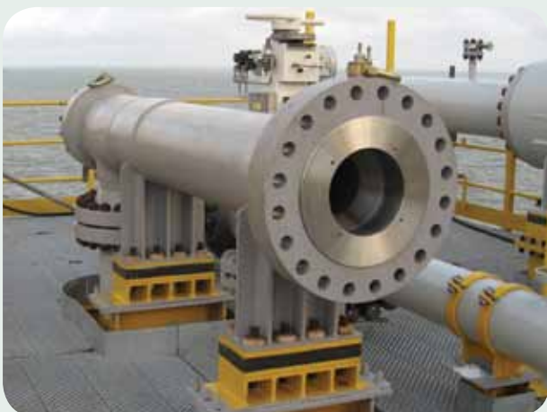
Transvac Patented Ejector boosted production by 15% using Compressor recycle gas
